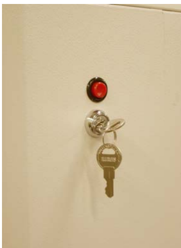
Figure 9. Security Key on side of Liquefier.
